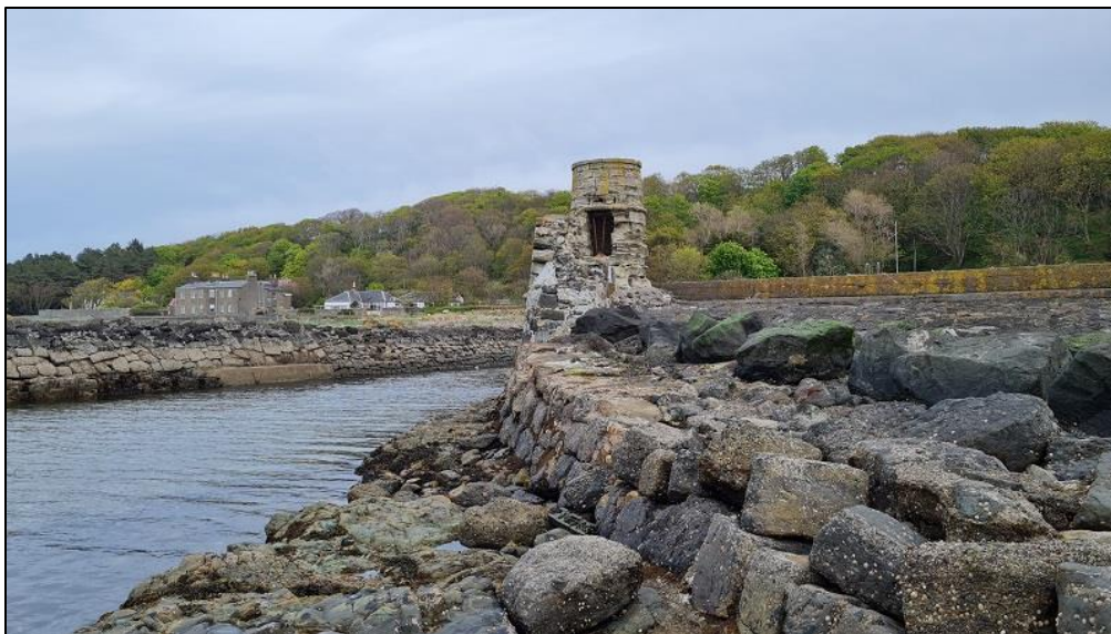
Figure 11c: W Breakwater E , Masonry Exposed at Low Tide
