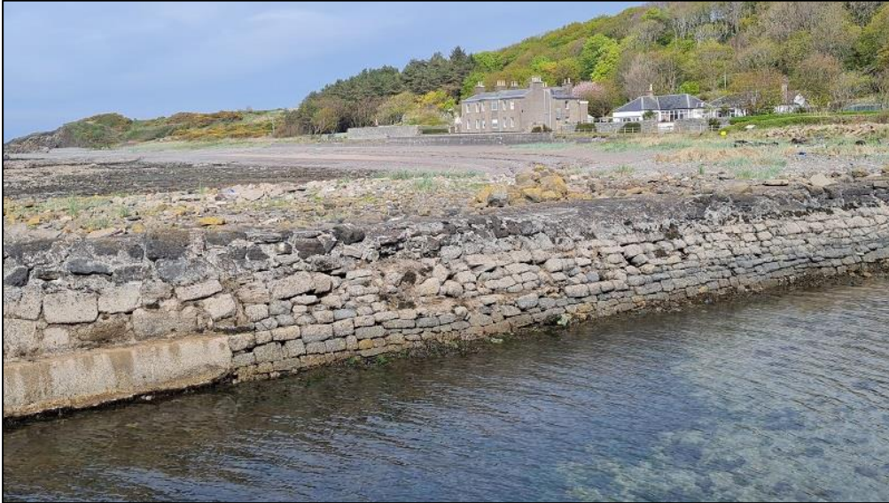
Figure 11a: Detail of Central Portion, North Breakwater D , Showing Variation in Masonry
