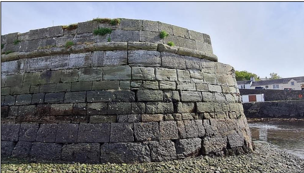
Figure 6b: Terminal of Quay Wall B1 Fully Exposed at Low Tide
