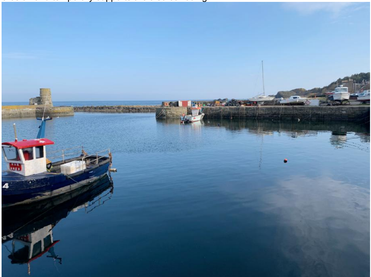
Normal High tide water level rises to the lower coursing of the sandstone on harbour walls
