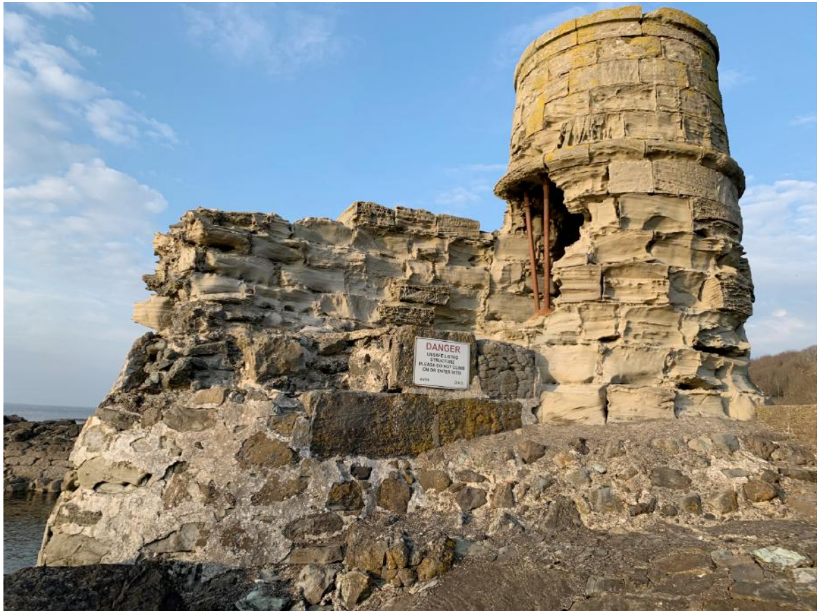
Condition of the Lighthouse structure and occulting wall has deteriorated badly with major erosion and temporary supports are also corroding
