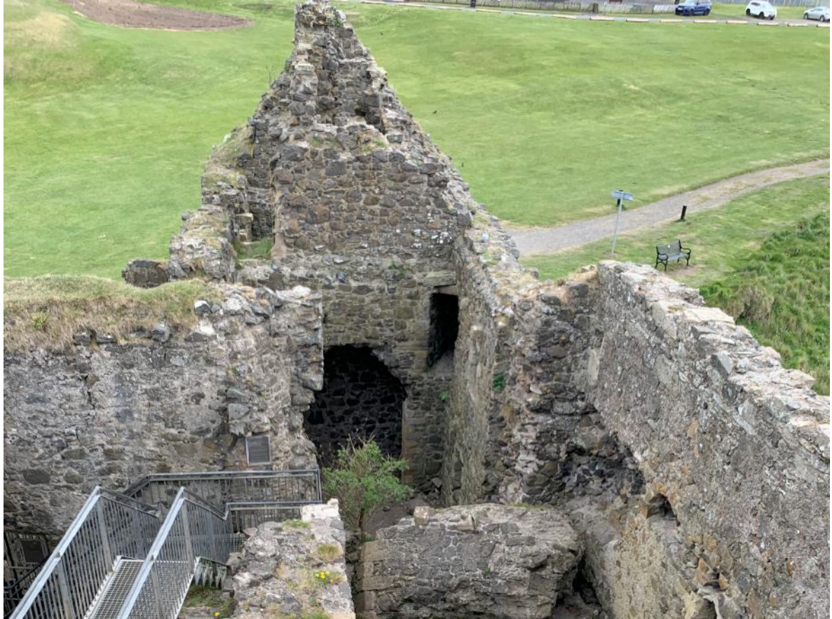
South building some loose stones on gable and wall-head require re-bedding
