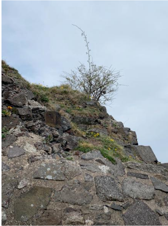
vegetation roots affect high level masonry
