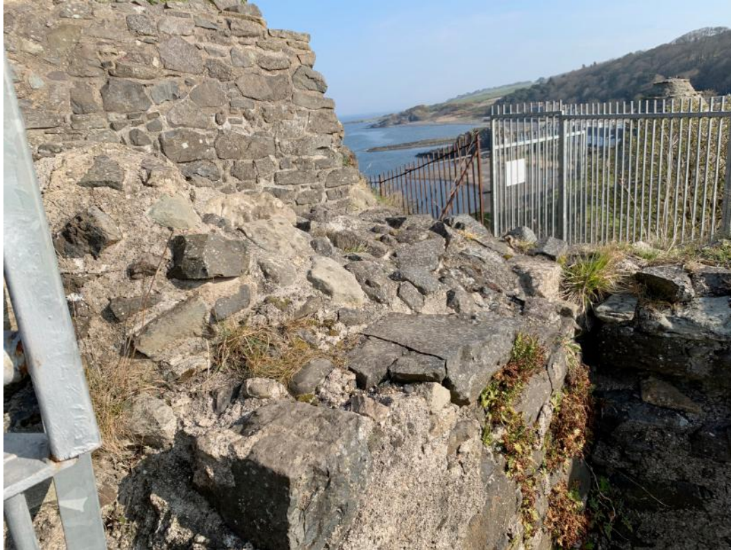
Corroding metal fencing at location frequently climbed for unauthorized access and some loose bedded stone – risks of falling and injury
