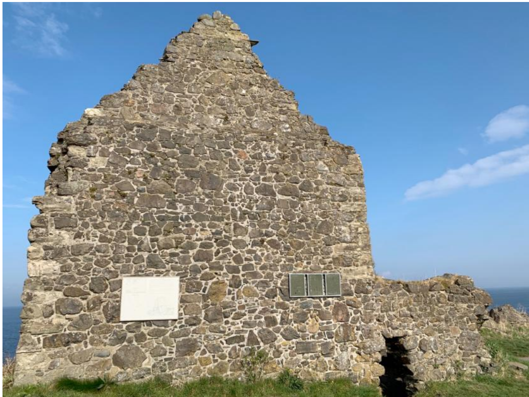
Interpretation boards have been bleached out by the sun and position on the wall is too
