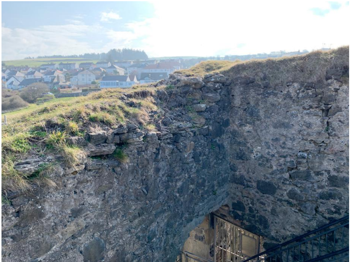
loose stones at turfed wall-head on South building and crack in masonry of inner gable
