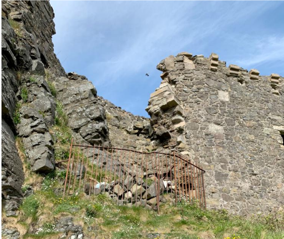
Fall of stones on West wall with some erosion of mortar and other loose stones
