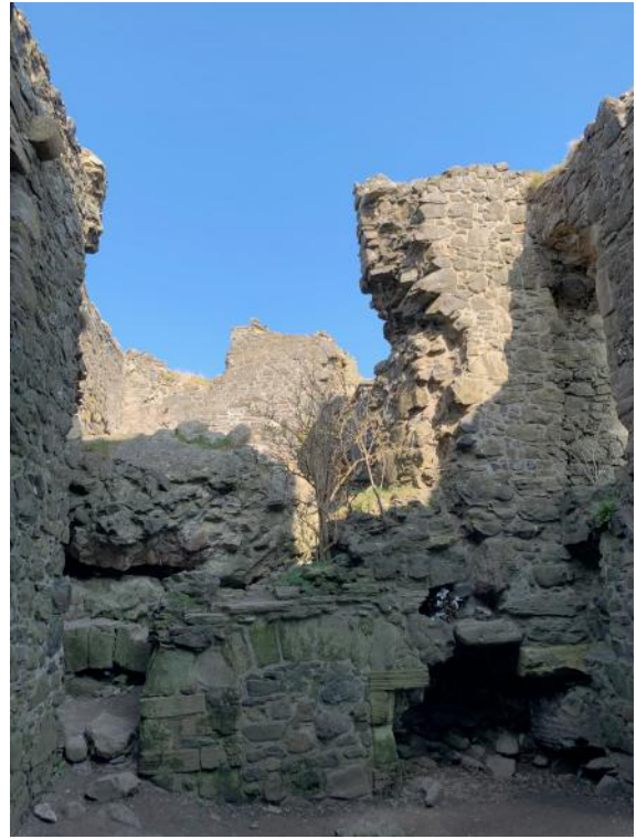
some loose masonry has fallen out of walls tree roots growing out of masonry
