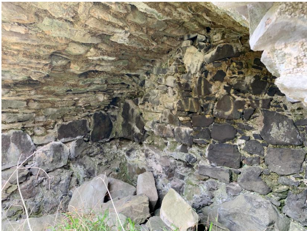
Lower tower arches masonry generally sound, some erosion of mortar
