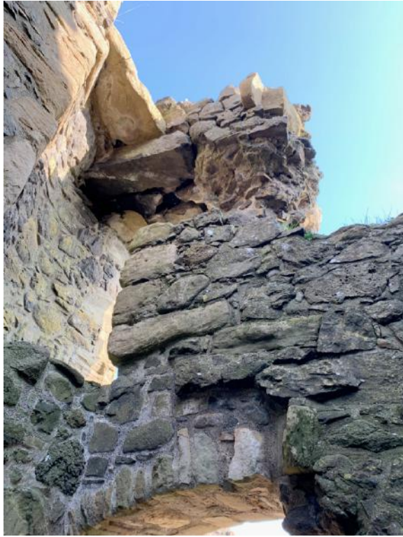
Crack in high level lintel High level eaves stone loose
