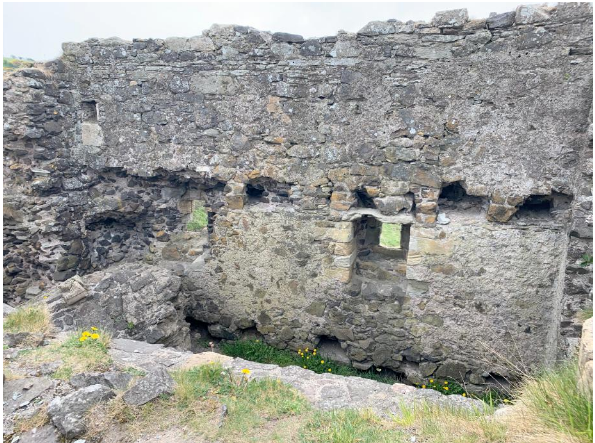
South building eaves stones loose in places
