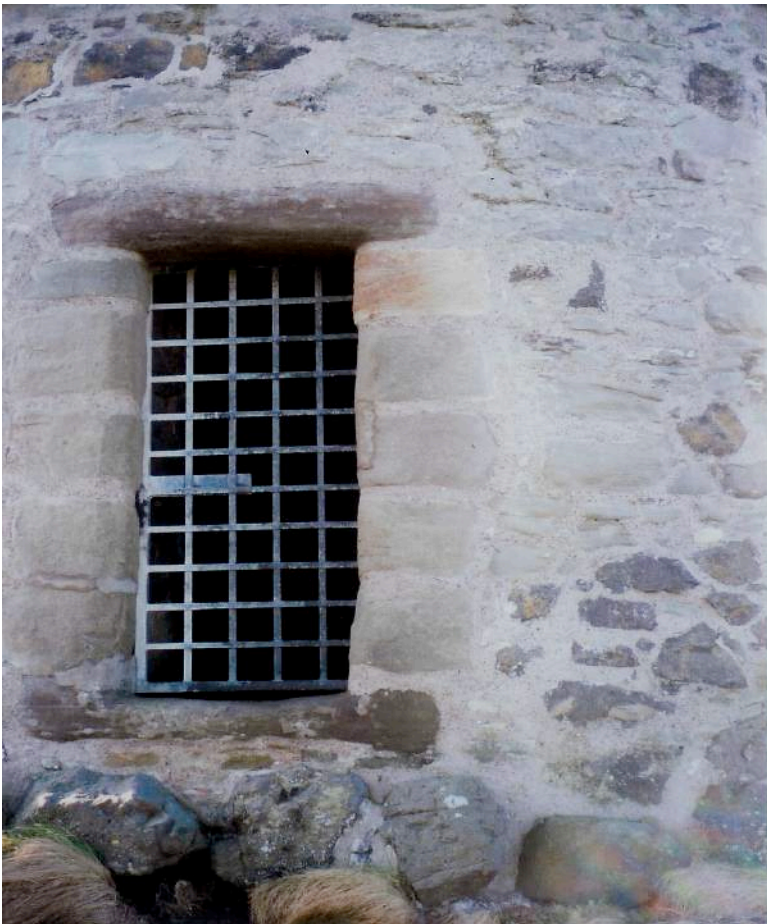
Fig 26: The new metal door and the new rendering of lime mortar and local shingle
