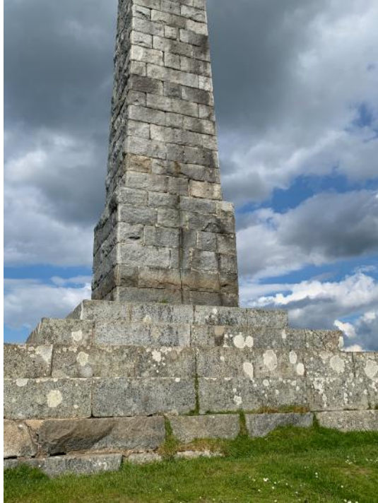
Plinth steps have some vegetation growing in joints
