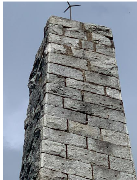
Upper mortar and joints poor and localised damage of some stones
