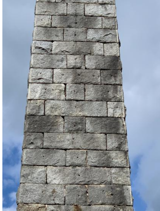
old fixing holes of lost conductor tape and scaffold fixings, to re-use and fill
