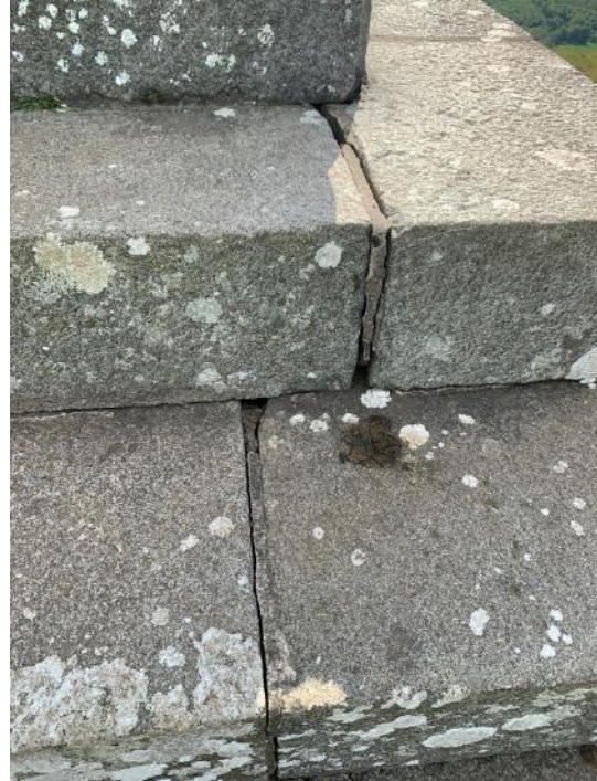
Mortar poor on steps top and face
