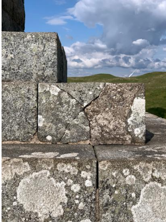
Stepped plinth with cracked stones And open joints
